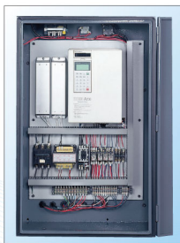
▲ Electrical box & inverter
